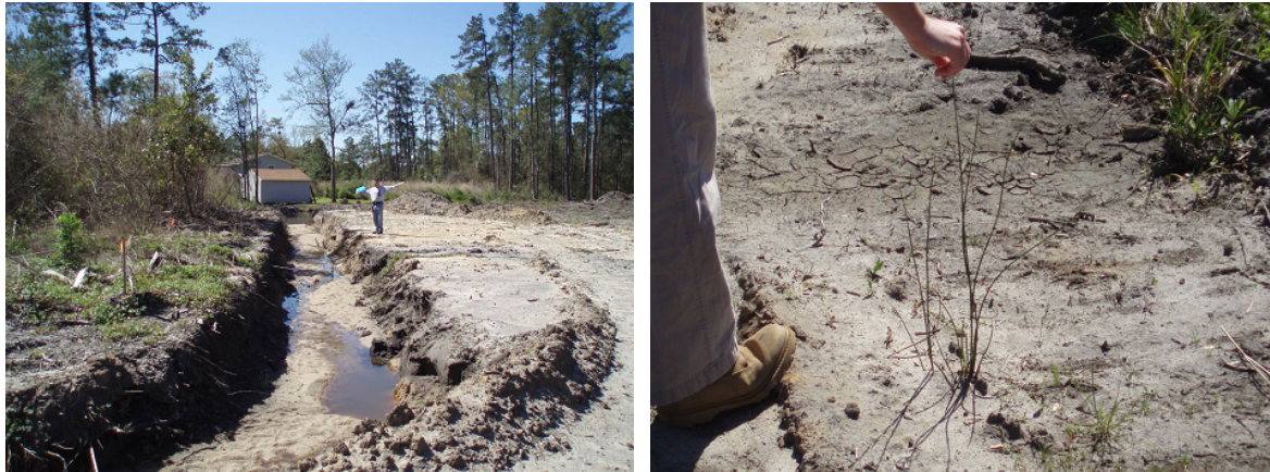
Figure 15. This small headwater stream in Conway, SC (left) once flowed through the middle of this recently graded development site. The stream was recently “relocated” to the property boundary, as evidenced by the remaining wetland plants (like the wetland rush shown in the photo on the right) emerging from the bulldozed earth.
